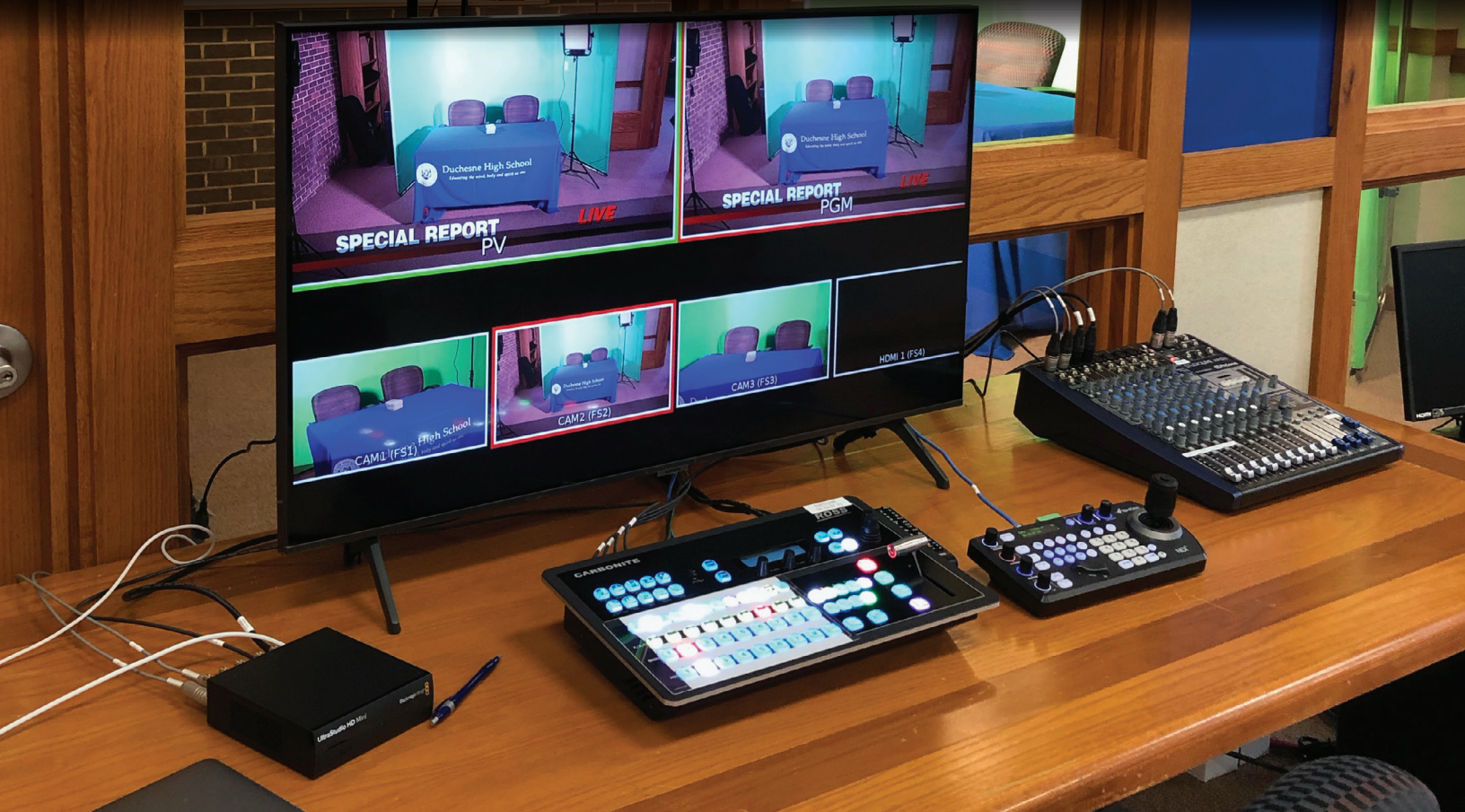
The switcher, camera controller, monitor, and audio board installed in Duchesne's new television studio as a part of 2022's Fund Our Future effort.
